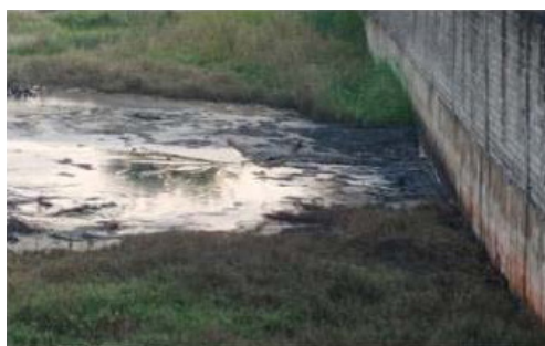
Figure 4.3: Leakage of liquid waste outside the boundary wall of the CBWTF
